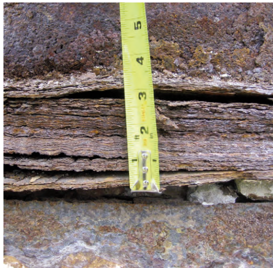
Fig. 5. Roanoke Building, Chicago, 1915 and 1925, corroded beam flange at 37th floor, 2005.
