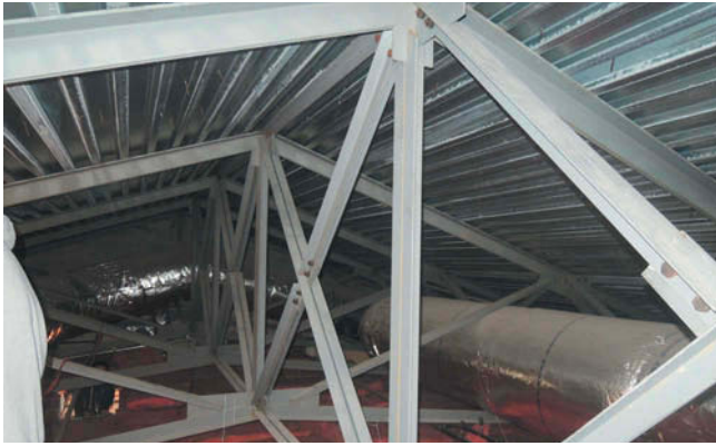
Lose-fitting and displaced insulation in attic.
