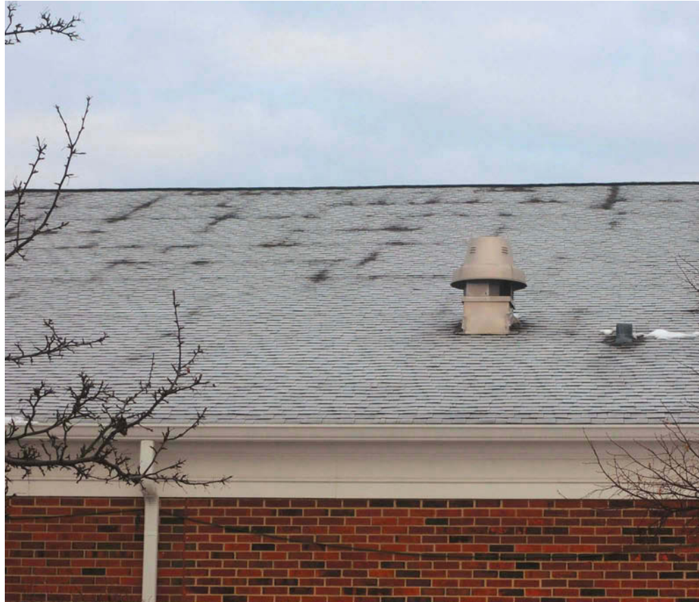
Patterns of frost-melt on roof surface.
