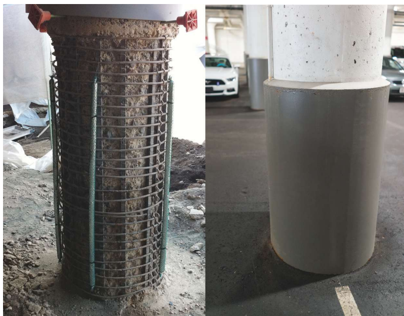
Fig. 7: Column jacket repairs during construction (left) and five years after rehabilitation (right)
