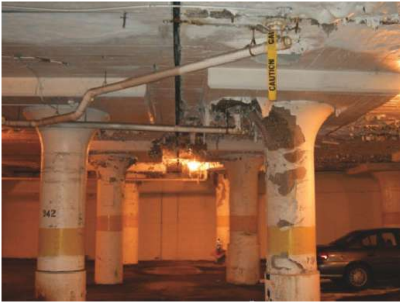
Fig. 3: Representative conditions at underside of track deck before rehabilitation
