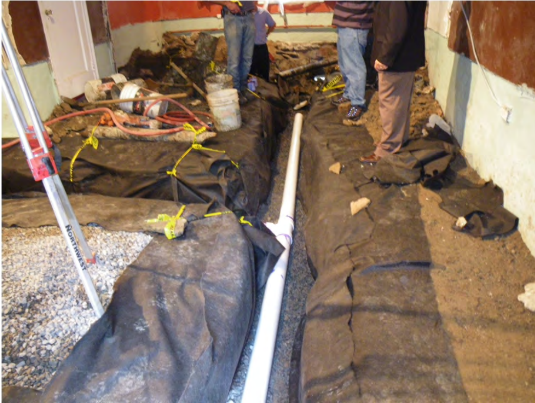
Subslab drainage system being installed as part of a water leakage repair project.
